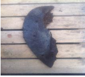
A quarter of the rotten baseboard !!
