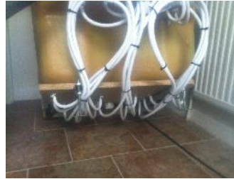
The new baseboard and system !
