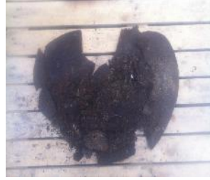
This is what was left of the baseboard which whilst the bath was being removed fell off !
